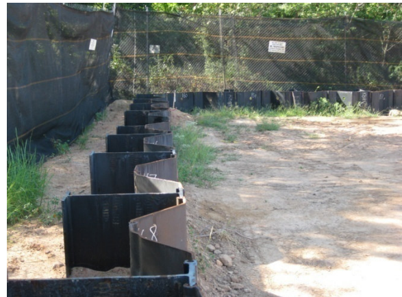
PZC-13 steel sheet piles driven with wide flange beams and extruded connectors
