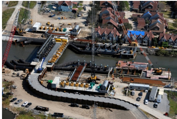
Aerial view of 17 th Street Canal during construction shows the 425-ft sheet pile-closed cell flood wall.
